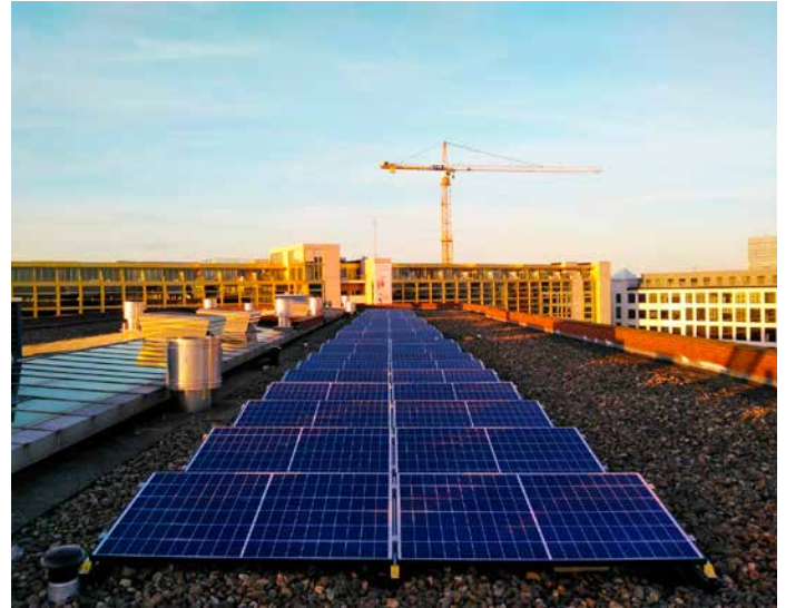
Solar panels Regentekwartier, Eindhoven
