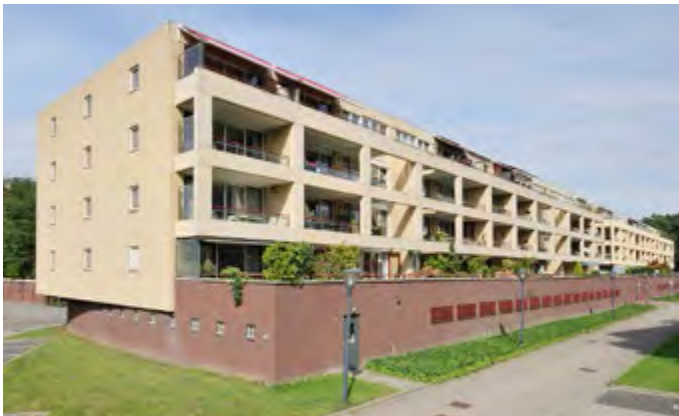
CBRE Dutch Residential Fund - Installment of LED lights and movement sensors, Hofwachter, Hofburg and Hofmeier in Geldrop
